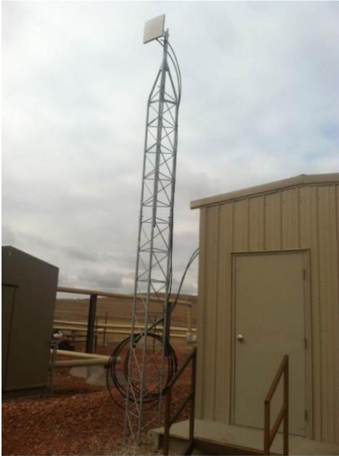
Mercury subscriber installed at oil well site
