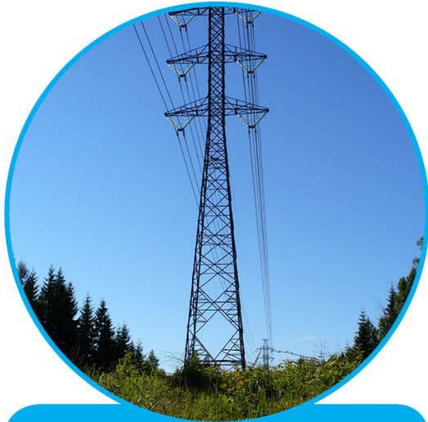
Electricity Transmission & Distribution
