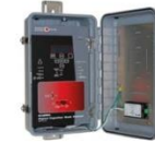
8 kV Capacitor Bank w/ M6280 Controller
