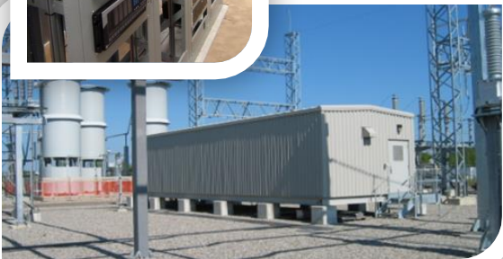
New Protection, Control & Telecom Building
