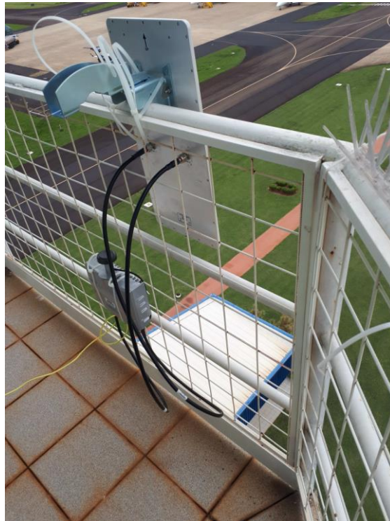
Figure 4: Antenna and Radio installation pointing to the runway.
