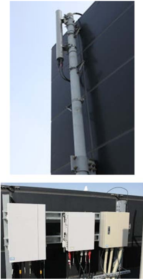
Figure 3. Base stations and antennas for rooftop installation (Source: UQ)
